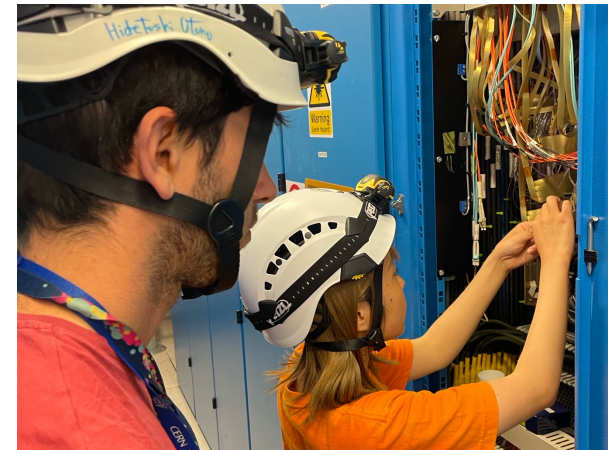
RX plugin replacement in the service cavern
